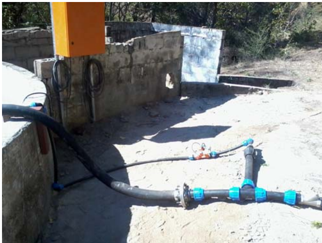
Tailings return water system
